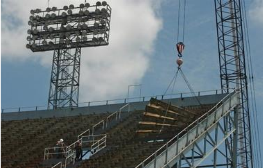
Because of structural problems that were too costly to repair, the Legion Field upper deck was torn down in 2005. (Joe Songer/jsonger@al.com)
