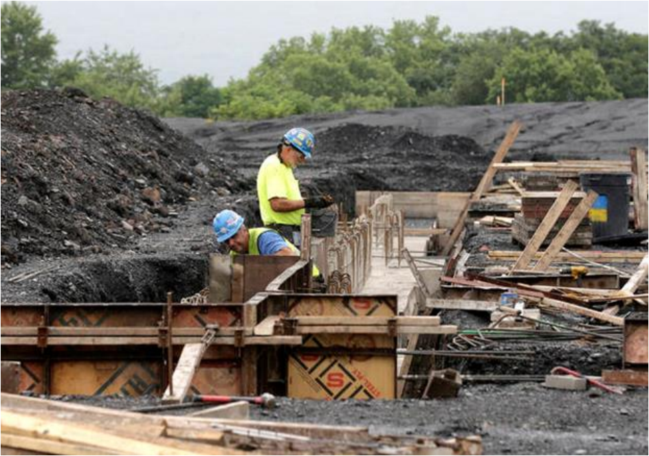
Contractors work on part of the foundation for the new Wilkes-Barre Area consolidated high school Monday foundation Bill Tarutis | For Times Leader
