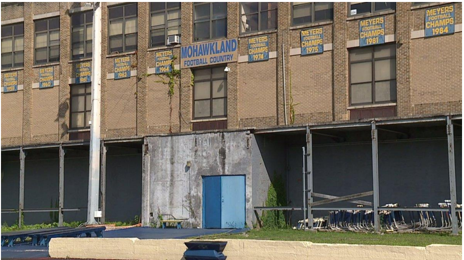
High School Stadium in Wilkes-Barre Closed for Repairs
