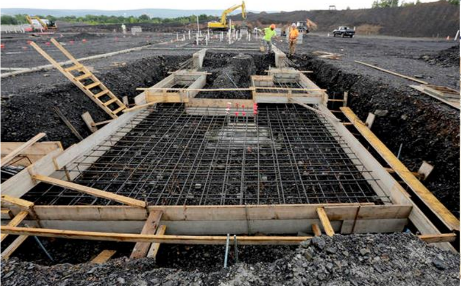
The base of an elevator shaft awaits concrete pouring on the construction site of Wilkes-Barre Area's consolidated school. (Mine Shaft High) Bill Tarutis | For Times Leader
