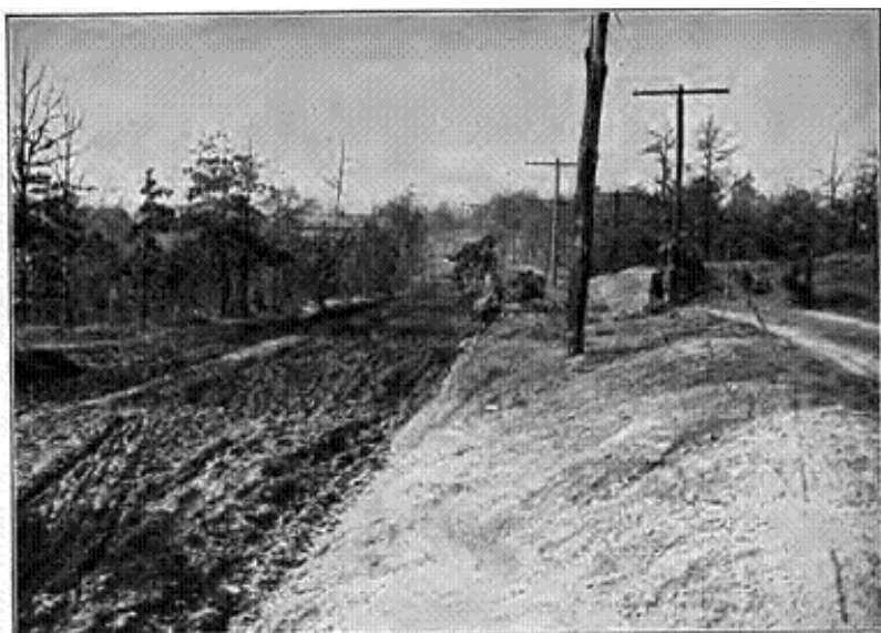
A ROAD BEFORE IMPROVEMENT
