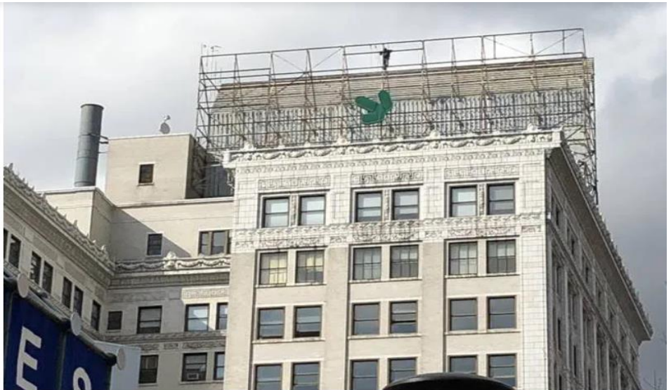
The downtown Wilkes-Barre skyline changed Friday afternoon when workers removed the last piece of the Citizens Bank sign from atop the 14-story building at the intersection of South Franklin and West Market streets. The building, designed by Chicago architect Daniel Hudson Burnham in 1911, was home to the Miners National Bank, the United Penn Bank and the Mellon Bank. The Citizens Bank moved out in February 2013. By then it had been purchased by Citi Tower LLC. The more than century-old high-rise has been remade into luxury apartments and renamed The Bank. Jerry Lynott | Times Leader
